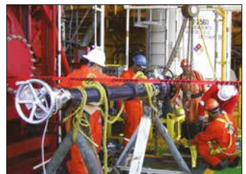
▼ CHT2000 hot tapping offshore application.
