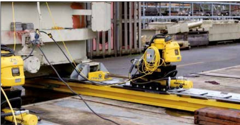
▼ A custom hydraulic Low-Height Skidding System will provide the maintenance team with the ability to maneuver and transport transformers with physical access limitations.
